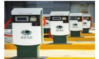
充電站 Charging Station
