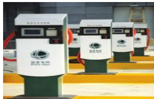
充電站 Charging Station
