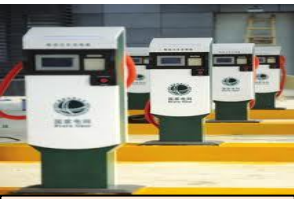
充電站 Charging Station
